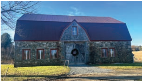
6. We finished a project to stabilize the Stone Barn Farm in Bar Harbor, replace the roof and roof bracing, and reconstruct the rear portion of the barn (though it looks nearly the same!). In coming years, we will continue to make important improvements to the land and buildings to increase accessibility and make the Stone Barn Farm preserve an even better community asset.
