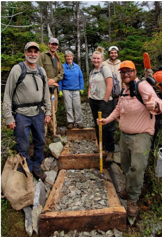
9. MCHT staff, seasonal crew members, and volunteers added two sets of stone steps at Boot Head Preserve on the Bold Coast. The preserve has soft, peaty soils, and, with increased visitation at the preserve, it's become necessary to harden added sections of Boot Head's trails. Harvesting and transporting lumber and heavy stones is quite labor intensive! Visitors can help protect fragile soils by keeping the trail tread narrow and using bog bridging and rock steps when provided.
